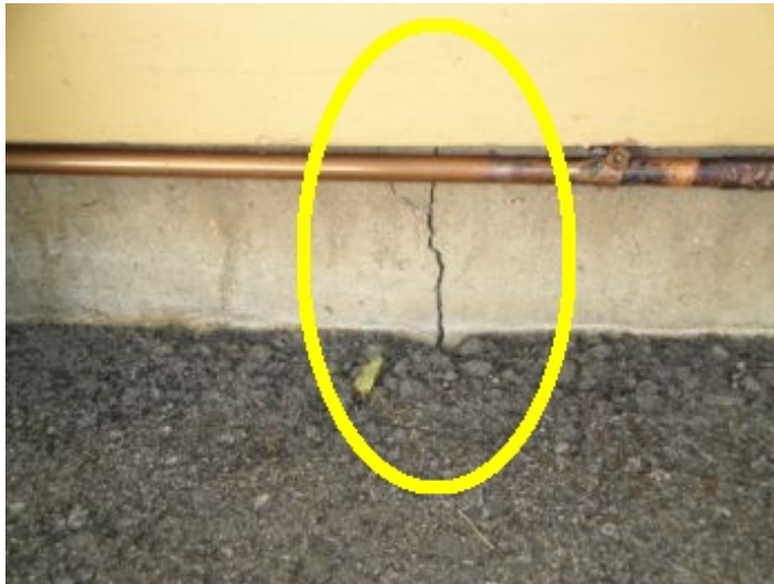
Small crack in the foundation wall, south side
