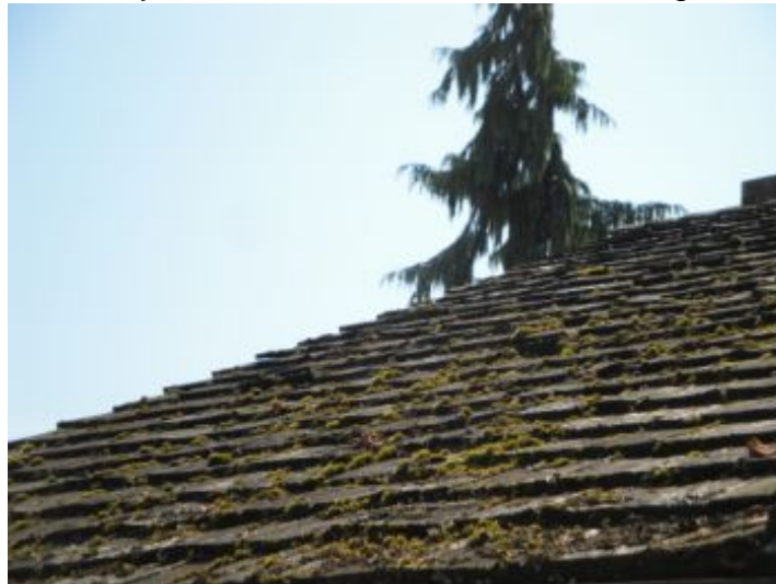
Extreme moss growth on roof
