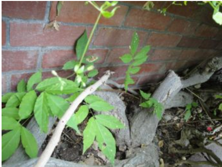
Vegetation is too close to the exterior
