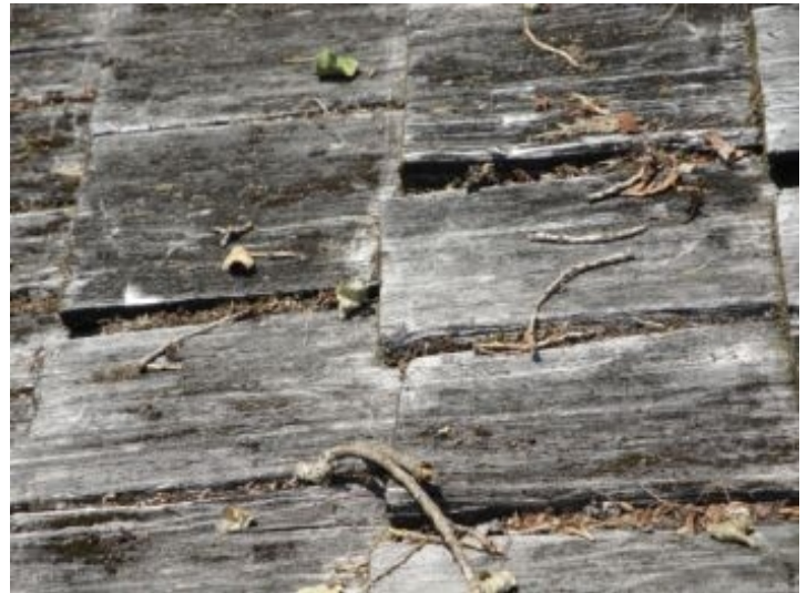
Damaged, old roof shingles
