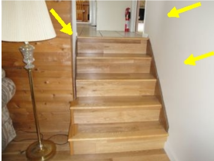
Missing hand rail up to kitchen, safety concern
