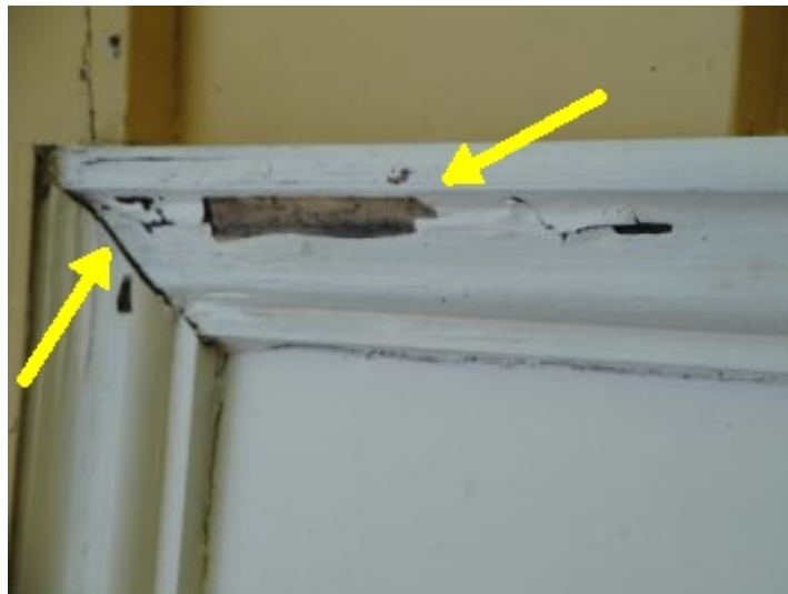
Wood rot on the garage door trim
