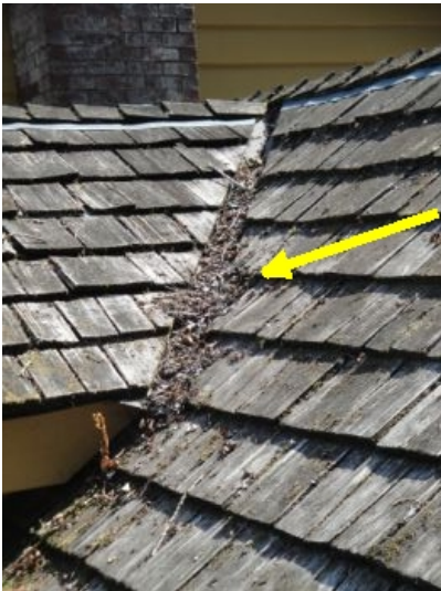
Debris in roof valley
