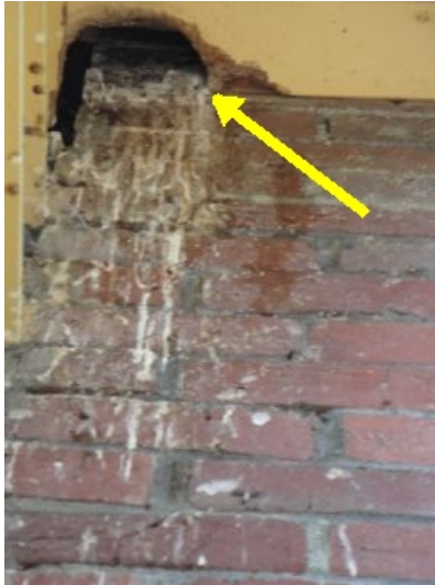
Soffit damage & evidence of nesting birds
